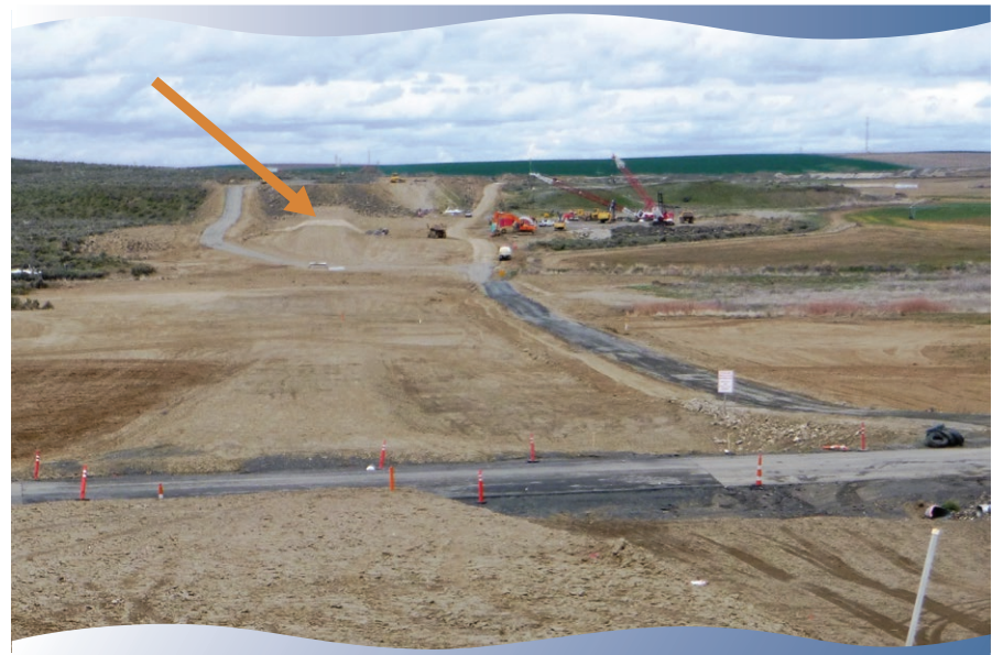
View from existing outlet structure of Lind Coulee Siphon No. 2 looking north across Lind-Warden road after completion of construction.
