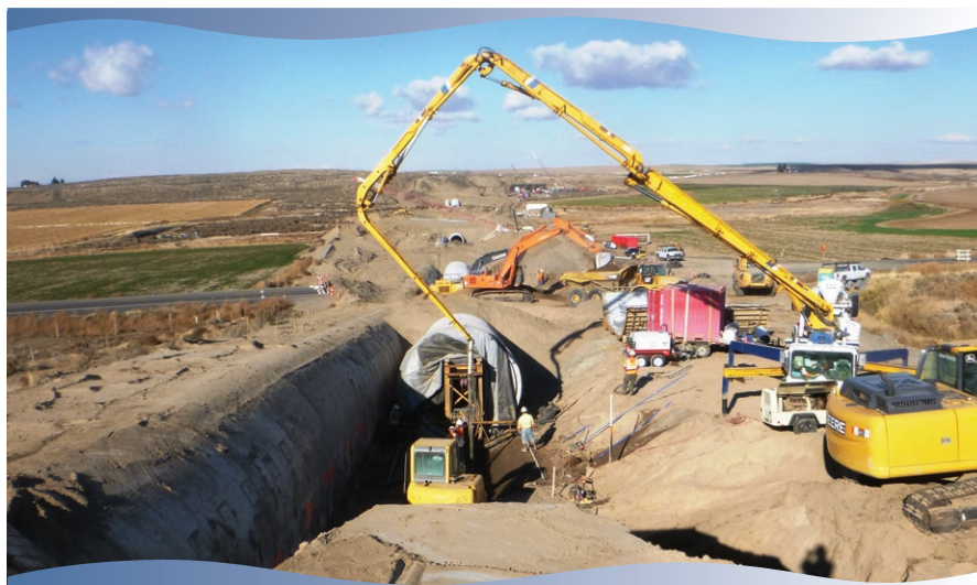
View from existing outlet structure of Lind Coulee Siphon No. 2 looking north across Lind-Warden road during excavation at road closure.
