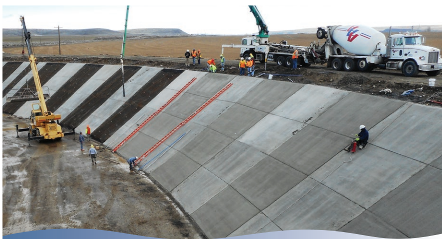
Concrete panels being poured on the Main Canal near F Road Northeast.
