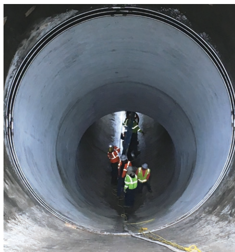
In late March, before the irrigation season began, ECBID staff conducted a walkthrough inspection tour of the Warden Siphon.
