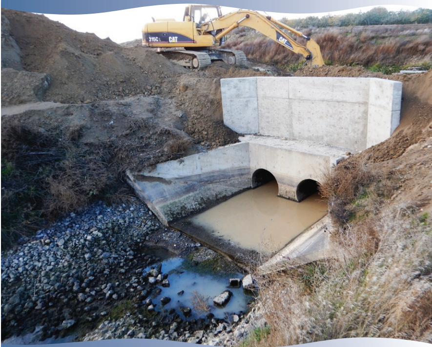
South Columbia Basin Irrigation District (SCBID) excavates the head of the WB5G Headworks after sink holes and separated pipe joints were discovered under the O&M road.
