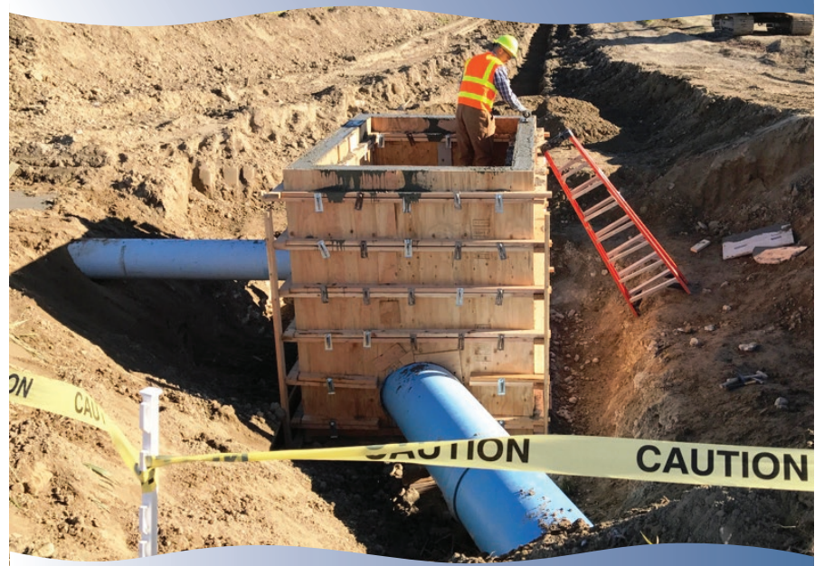
Quincy Columbia Basin Irrigation District (QCBID) completes a pipeline project at Blyth. This project entails adding a pipeline to a lateral in Block 85 that delivers to four farm units. There are multiple benefits to piping a lateral including reducing the cost of maintaining the lateral by eliminating the need to mow, spray, or control aquatic weeds, lessening the liability of a potential canal breach, allowing landowners more flexibility on the use of their land, and ultimately conserving water.
