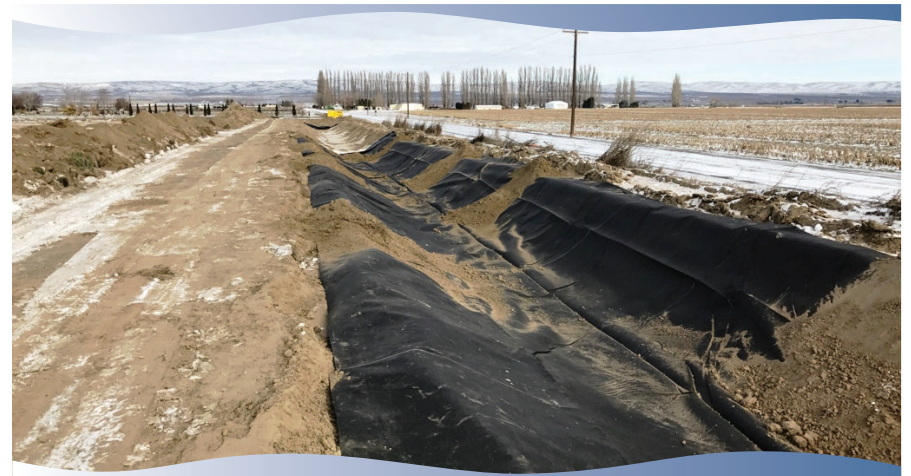
QCBID works on a canal lining project in the W33B lateral in Block 72 in Quincy section. Benefits of canal lining are similar to the pipeline project and include reducing the chance of a canal breach and conserving water by reducing the possibility of seepage.
