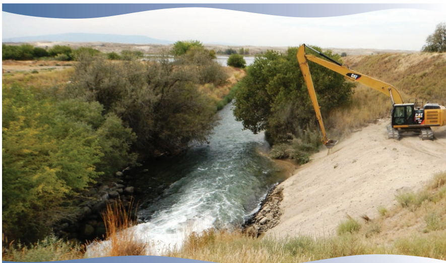
SCBID repairs an eroded bank on the PE16.4 Waste Way near its terminus.
