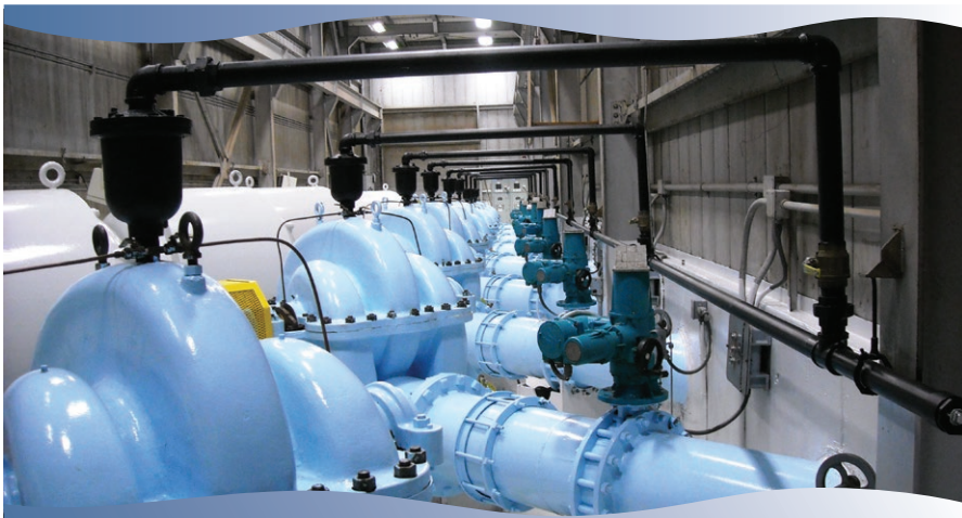
The Babcock pumping plant was recently repainted by the Quincy section crew.
