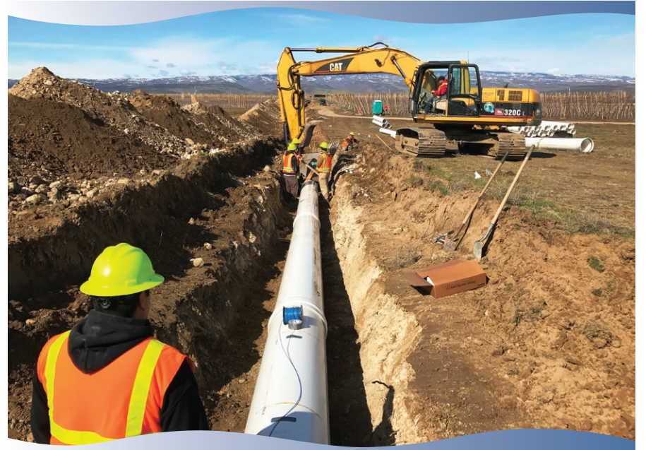
W44C7 Pipeline work, a landowner cost share project, done by the George section crew.
