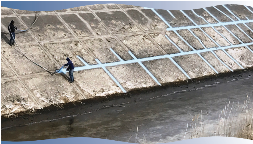
Two workers seal cracks with polyuria on the Main Canal. The work was contracted to Columbia Industrial Coatings, Inc. and 5,060 gallons of AquaLastic were applied.
