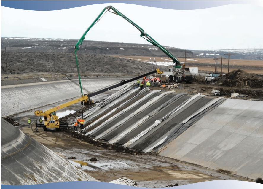
A view of panel replacement work on the Main Canal, contracted to West Company, Inc. 491 panels were removed and replaced throughout March.
