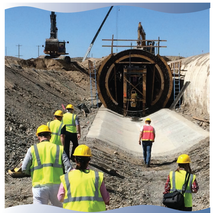
Members of the media get up close view of the Lind Coulee Siphon Construction.
