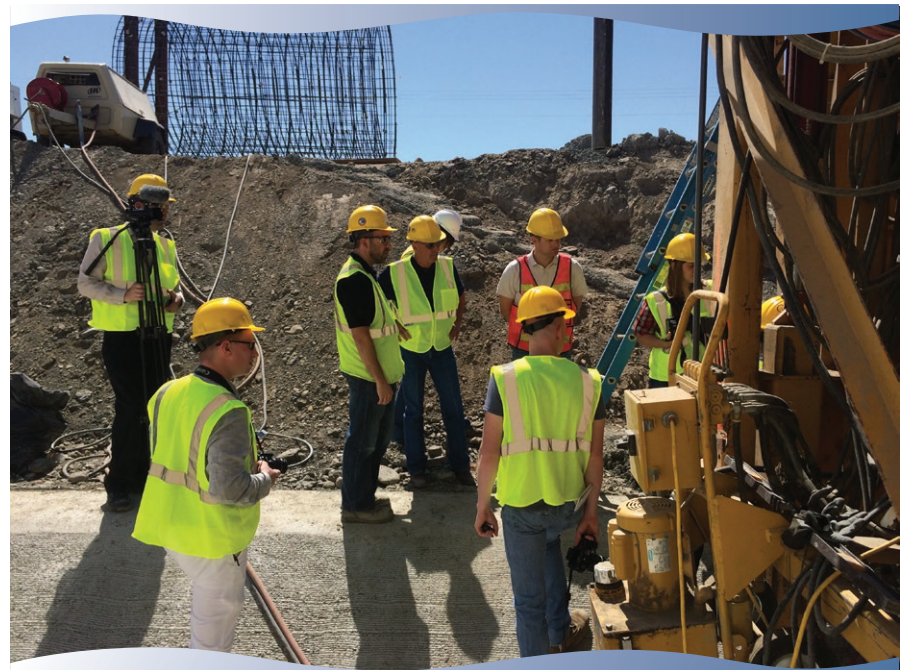
ECBID Development Coordinator Levi Johnson and members of the media at Lind Coulee Siphon Construction Site.
