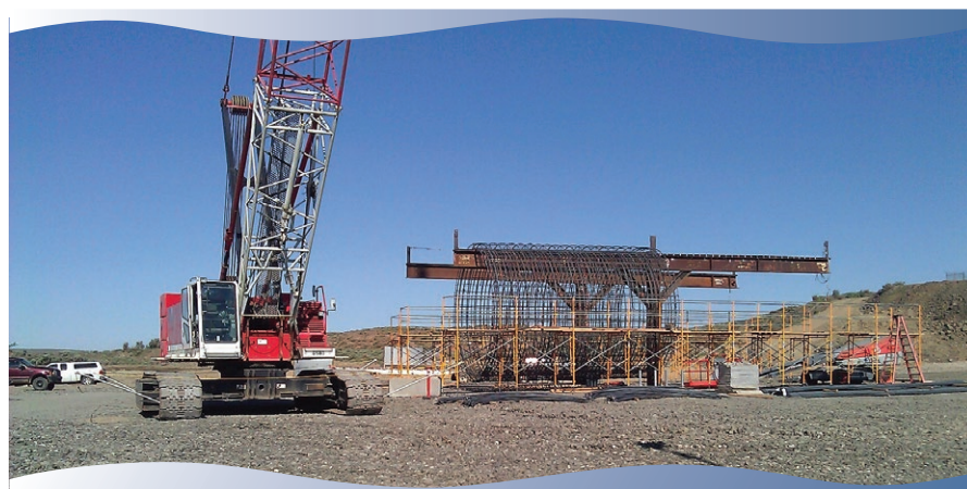
Rack used to assemble rebar cages which are then slid inside the moveable slip form.
