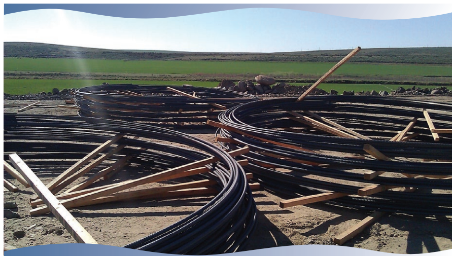
Stacks of heavy gauge rebar that will be formed into cages for siphon section construction.
