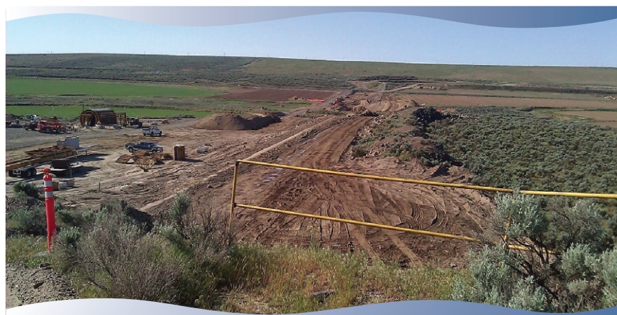
Pathway for Lind Coulee Siphon #2 with top of existing siphon just exposed.
