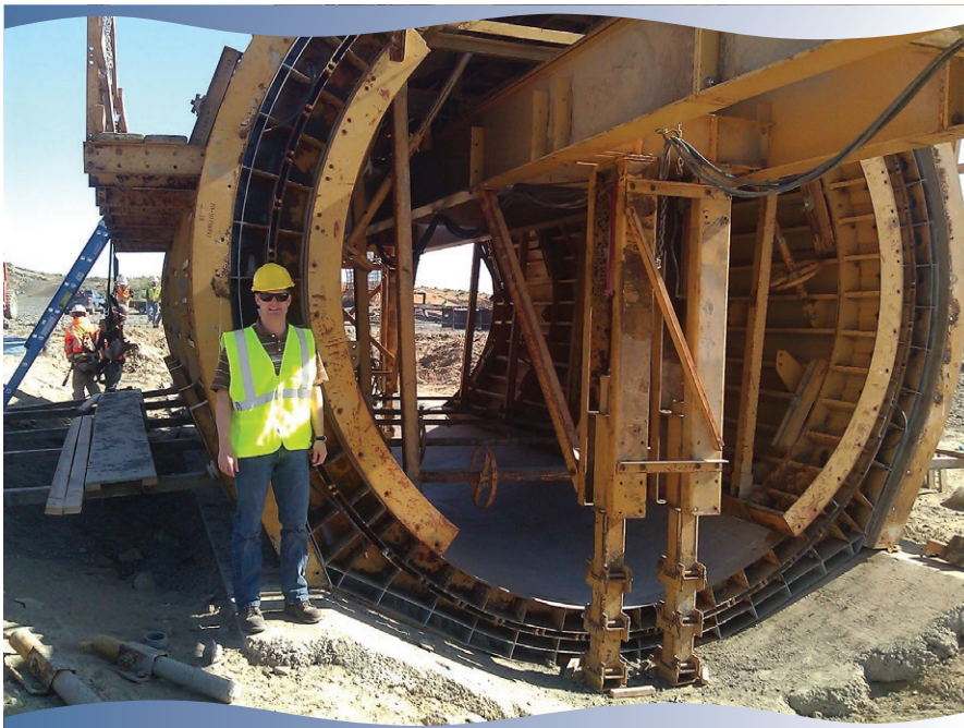
Levi Johnson, ECBID Development Coordinator, standing by the first test section for the Lind Coulee Siphon Project.
