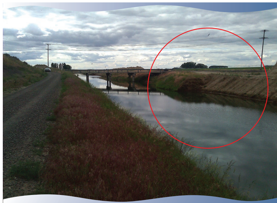
Canal expansion on Hatton Rd, southwest of Othello, waiting on new bridge construction.
