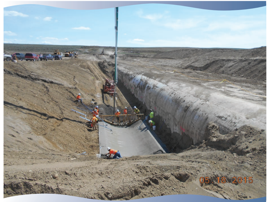
Foundation, or "rat slab," being placed on Lind Coulee siphon No. 2 next to original siphon barrel.
