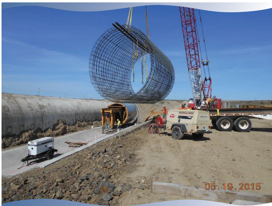
Placement of interior form and rebar cage for first new siphon barrel section on Lind Coulee No. 2.
