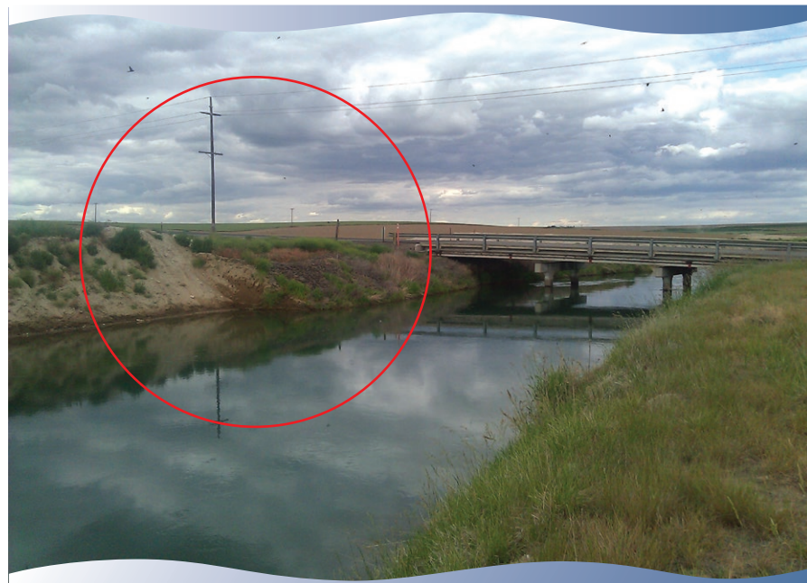
Continued canal expansion on Booker Rd., south of Warden, waiting on new bridge construction.
