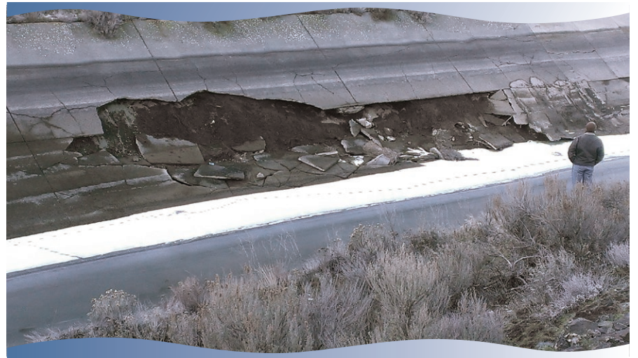
Panels needing replacement on the Main Canal upstream from Pinto Ridge Road.
